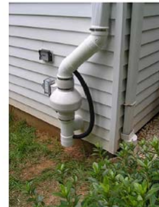
Photo 4 - System with Dilts by pass drain
